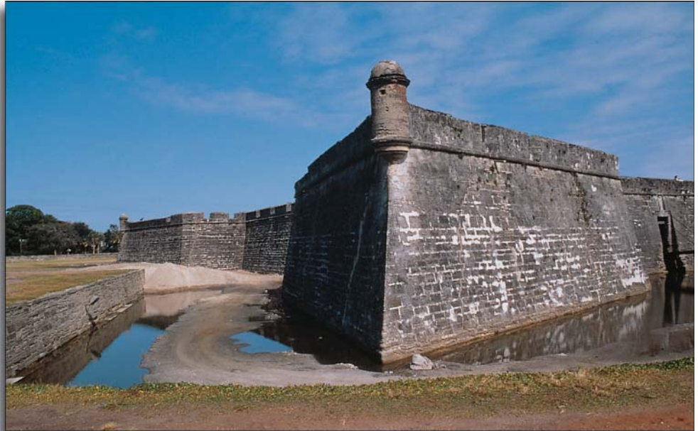
Cracks in the walls of Castillo de San Marcos, Florida were instrumented to determine their genesis and the best course for corrective action.
